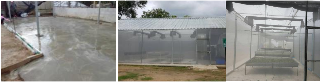
Fig 5. Rebuilding of mother plant net house of potato at Maehea (Dec 17-Jul 18).
