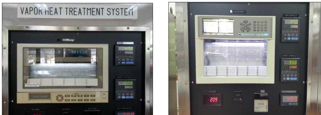
Figure 9 Recorder in the vapor heat treatment system
