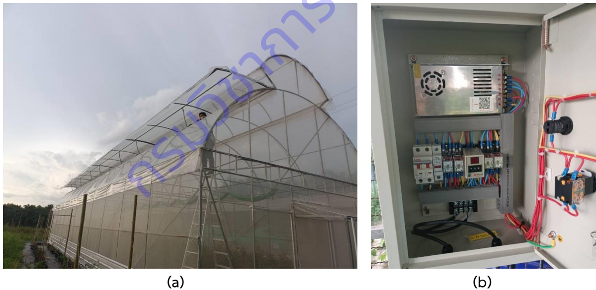
Figure 6.1-3 Development of hot air ventilation system when high temperature (a) the roof of the greenhouse can be opened to cool down by having another layer of insect nets inside (b) the roof opening and closing control cabinet
