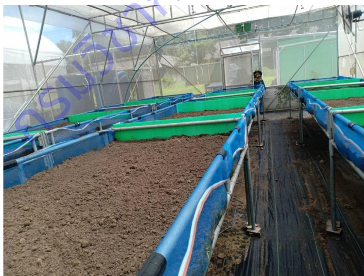
Figure 6.1-10 Installing cameras in greenhouses and installing a wifi system to support image processing.
