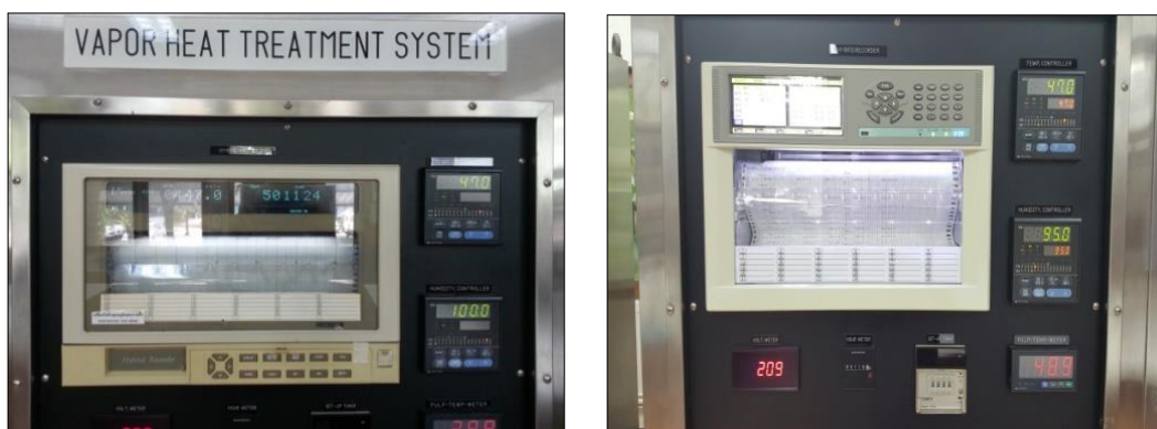
Figure 8 Recorder in the vapor heat treatment system
